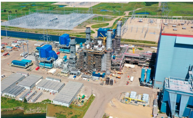
The Genesee Repowering Project is located on the west side of the power plant site. Once complete, the combined cycle facility will produce 1,338 MW of cleaner, reliable baseload electricity for Alberta.
