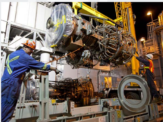
Two of Decatur Energy Center's three turbines were replaced during 2019 and 2020 maintenance outages, adding approximately 60 MW of additional capacity.
